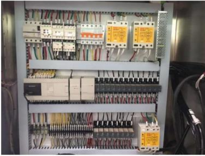
Control Box Mitsubishi,Schneider,CKD,Omron
